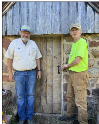
The outside of the spring house with the new door – David Mecklenburg and Duane Schmidt.
