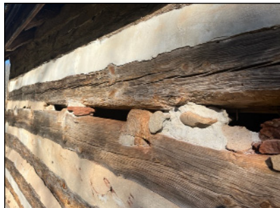
Missing chinking in the smoke house.
