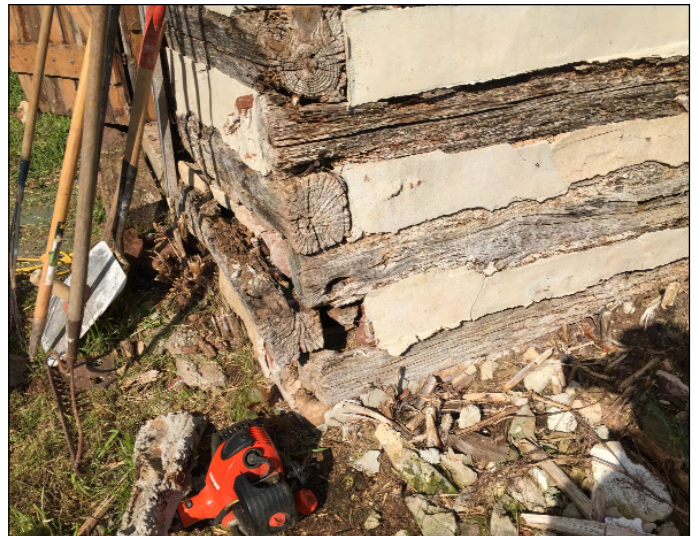
Smoke House Log Damage
