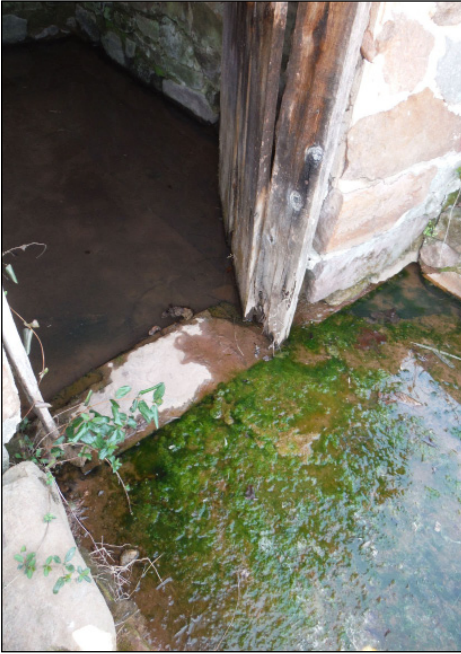
Prior to repair - damed-up water flow
