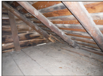
Critter chewed log rafter
