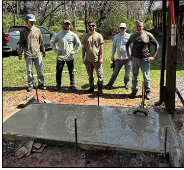
Access ramp poured at R&P Range. All part of our improving the accessibility at the chapter.
